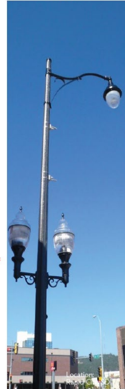
Figure 223: Decorative Light Fixture
