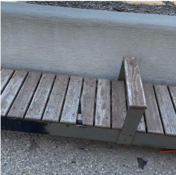
Damaged wood bench seat slats
