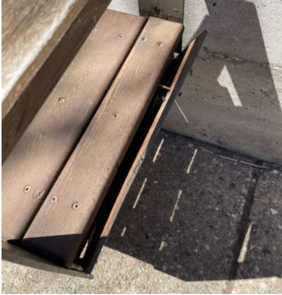
Cracked and loose metal on welded bench frame
