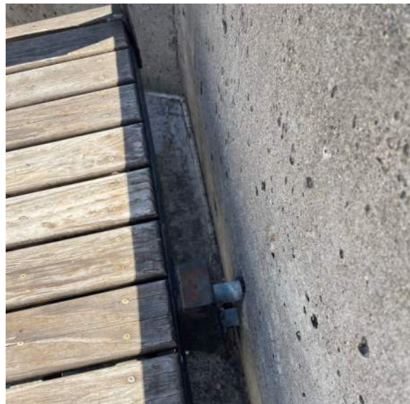
Failing bench structural support connections)
