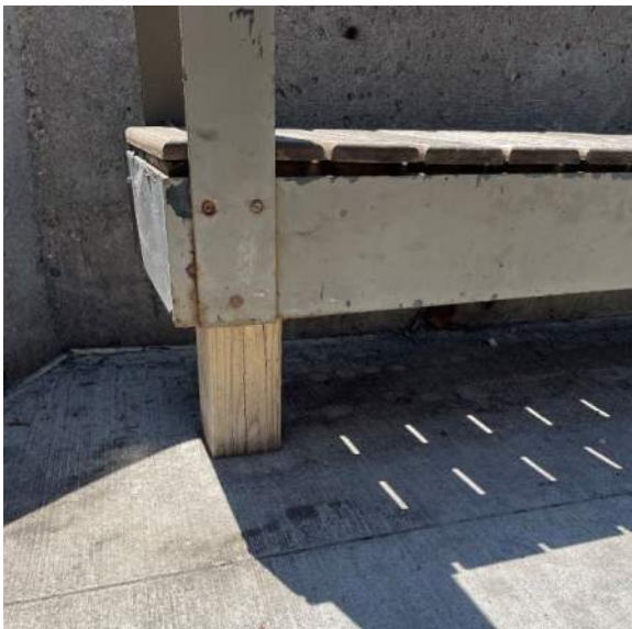
Failing bench structural support connections) (wood 4x4 post used to prop up bench)
