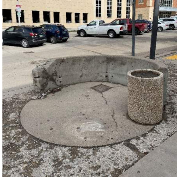
Missing bench and damage to / missing concrete structural shell
