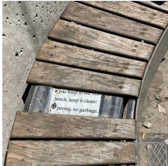
Missing wooden bench seat slats
